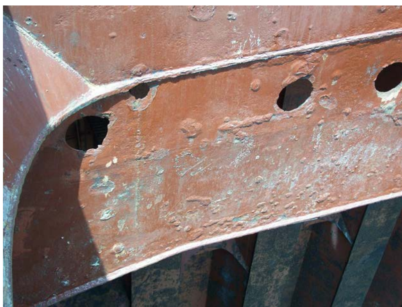
Photograph 2 Heavy corrosion of hatch coaming
