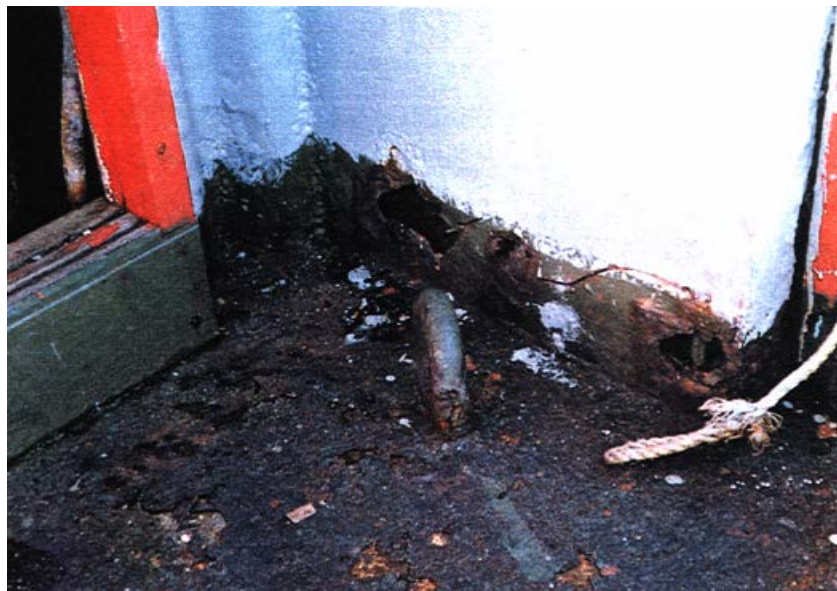
Photograph 1 Corroded accommodation house structure
