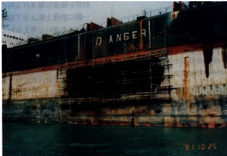
Photograph 2 Missing side shell structure (See Examples 4 and 5)
