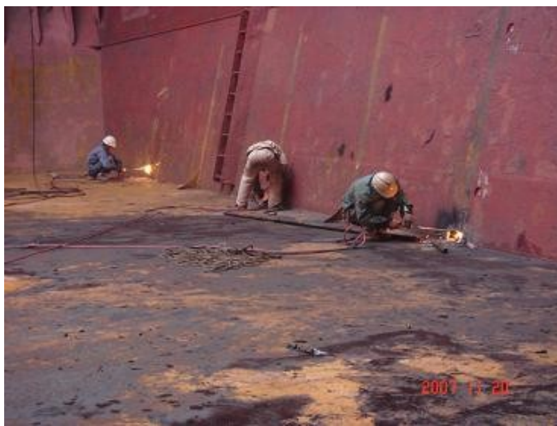
Photograph 1 Heavy corrosion affecting inner bottom plating
