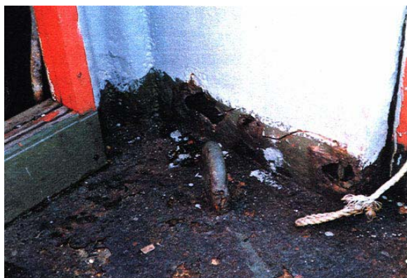
Photograph 1 Corroded accommodation house side structure
