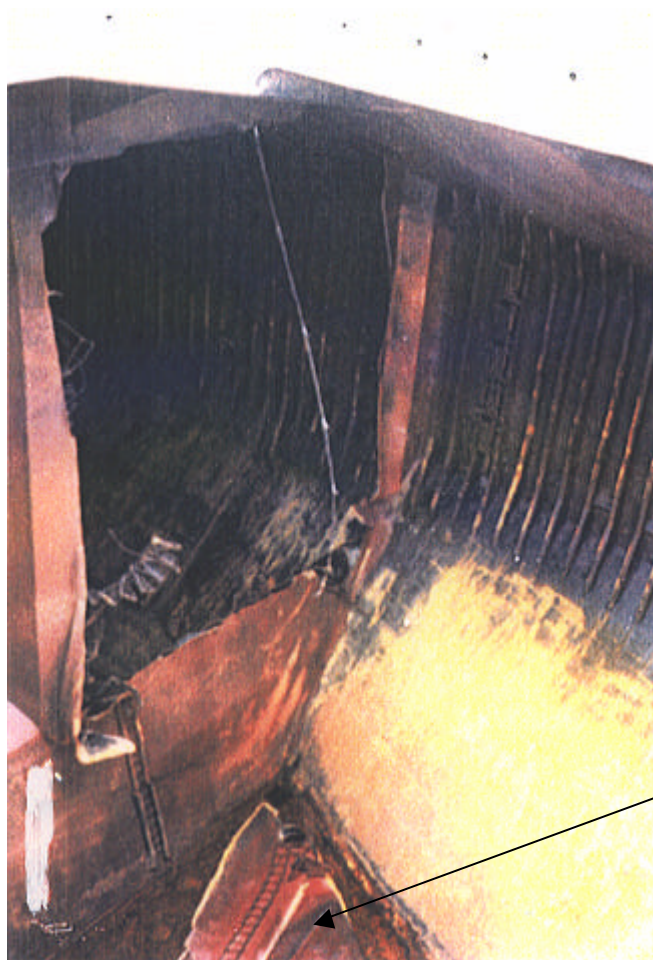
Photograph 1 Collapsed and detached transverse bulkhead
