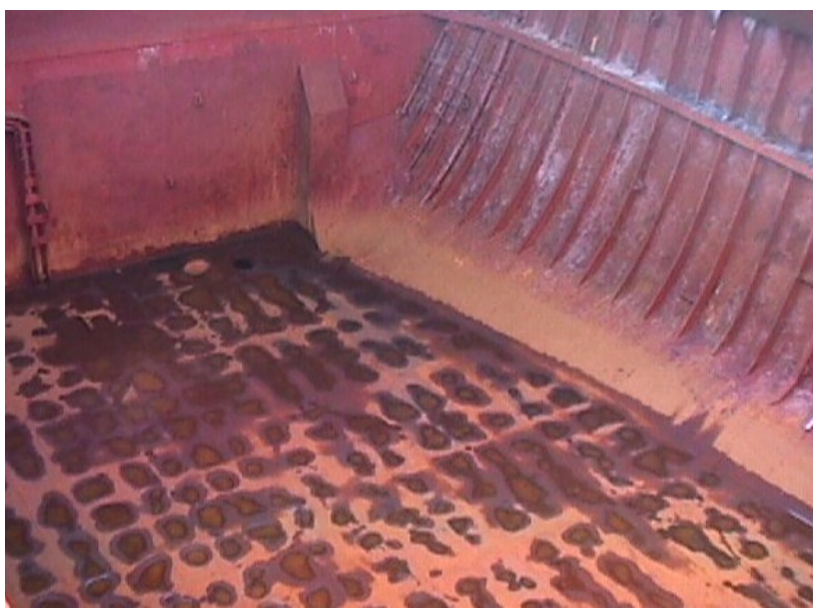
Photograph 2 Damaged inner bottom plating
